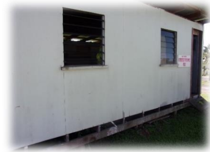
One example of Quick KAIZEN: The vacant wood house was renovated to store IPC consumables.
